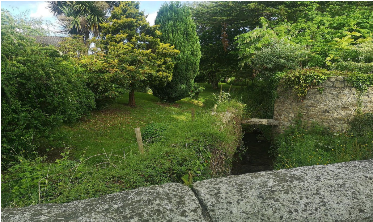
Figure 14.6: Image of Kilgobbin Road (Private Garden of 'Riverside') showing location of existing Historic Wall to be removed and reconstruct. A proposed defence wall will be located within the private garden.
