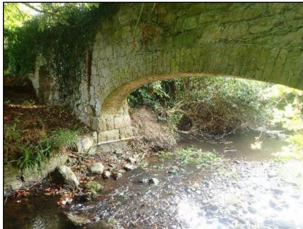
Figure 13.40: CH10 (ADCO 6) arched boundary wall located at the upstream end of the flood measure
