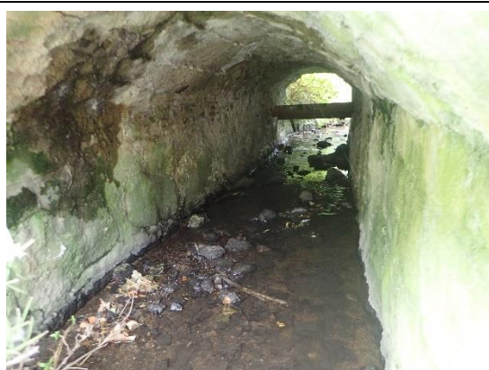
View along the northern barrel vaulted arch, showing the large boulder used to construct the bridge piers, and the later repairs to the vault
