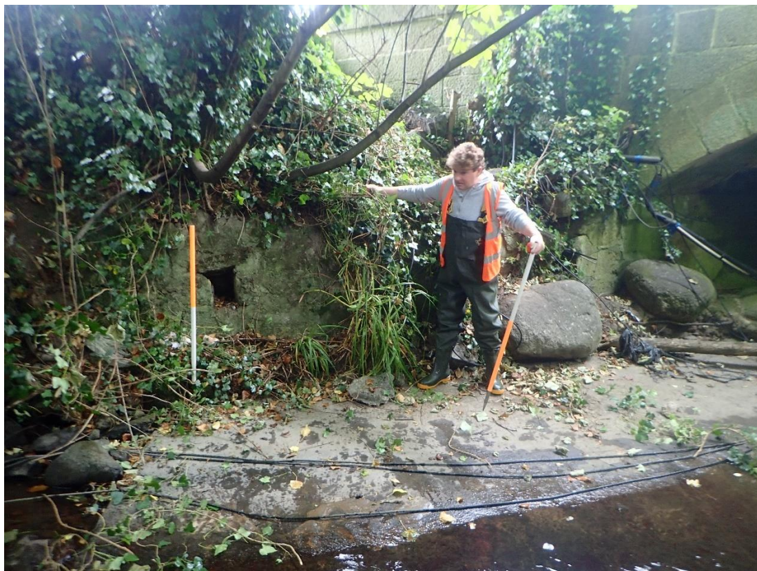
Plate 20: View of retaining wall upstream of and associated with Loughlinstown Bridge, ADCO 9. The riverbed at this point is covered in the stone apron that is also associated with the bridge.
