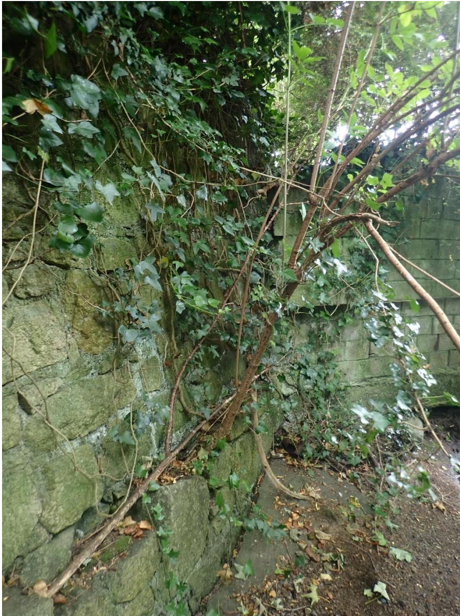
Plate 21: Expanse of breeze blocks to the right that replace stone wall to the left (ADCO 7), where the stone wall has collapsed or been removed.
