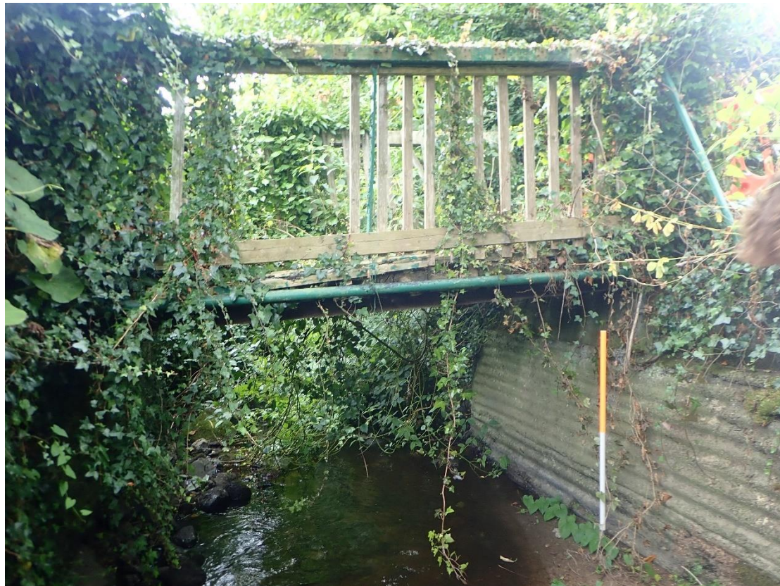
Plate 1: Footbridge is constructed on steel girders and has a light open timberwork parapet. The right bank underneath the bridge has been strengthened by the addition of a concrete pour
