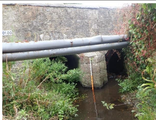
View from upstream at bridge arches and cutwater. Modern service pipes cross in front of the bridge
