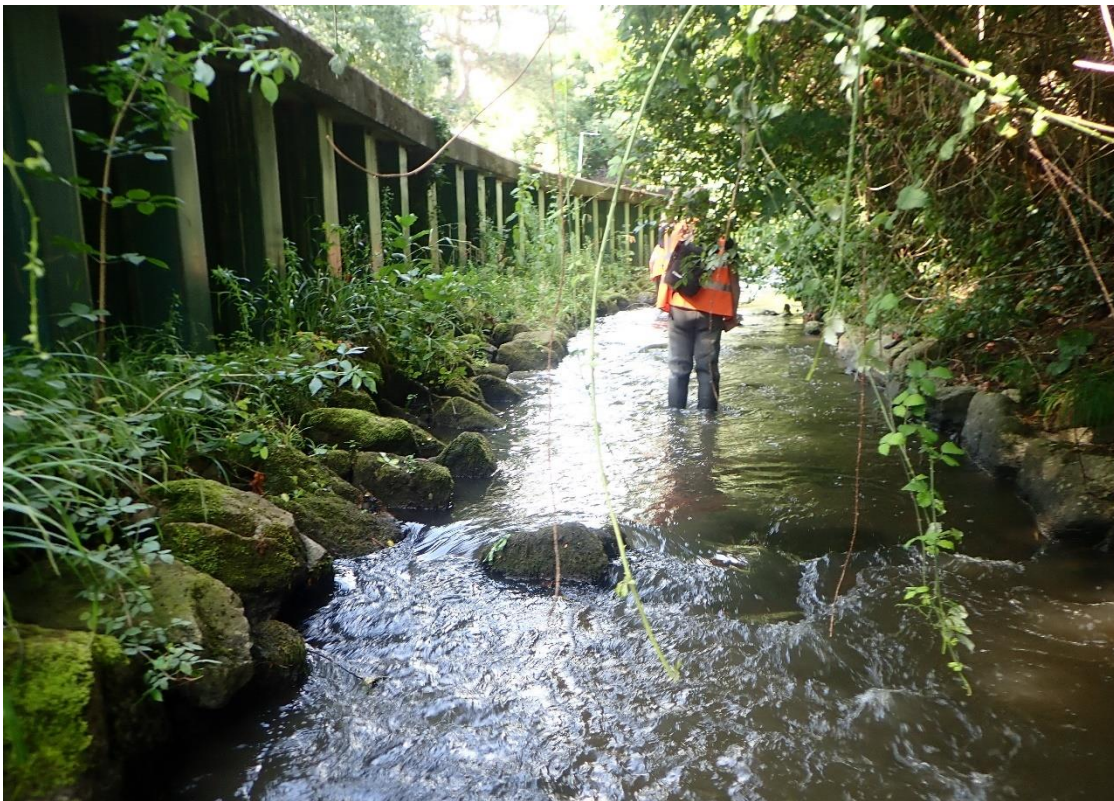
Plate 2: View looking upstream showing Larsen piling and rock armour protection that defines the right bank downstream of Shangnagh Bridge.
