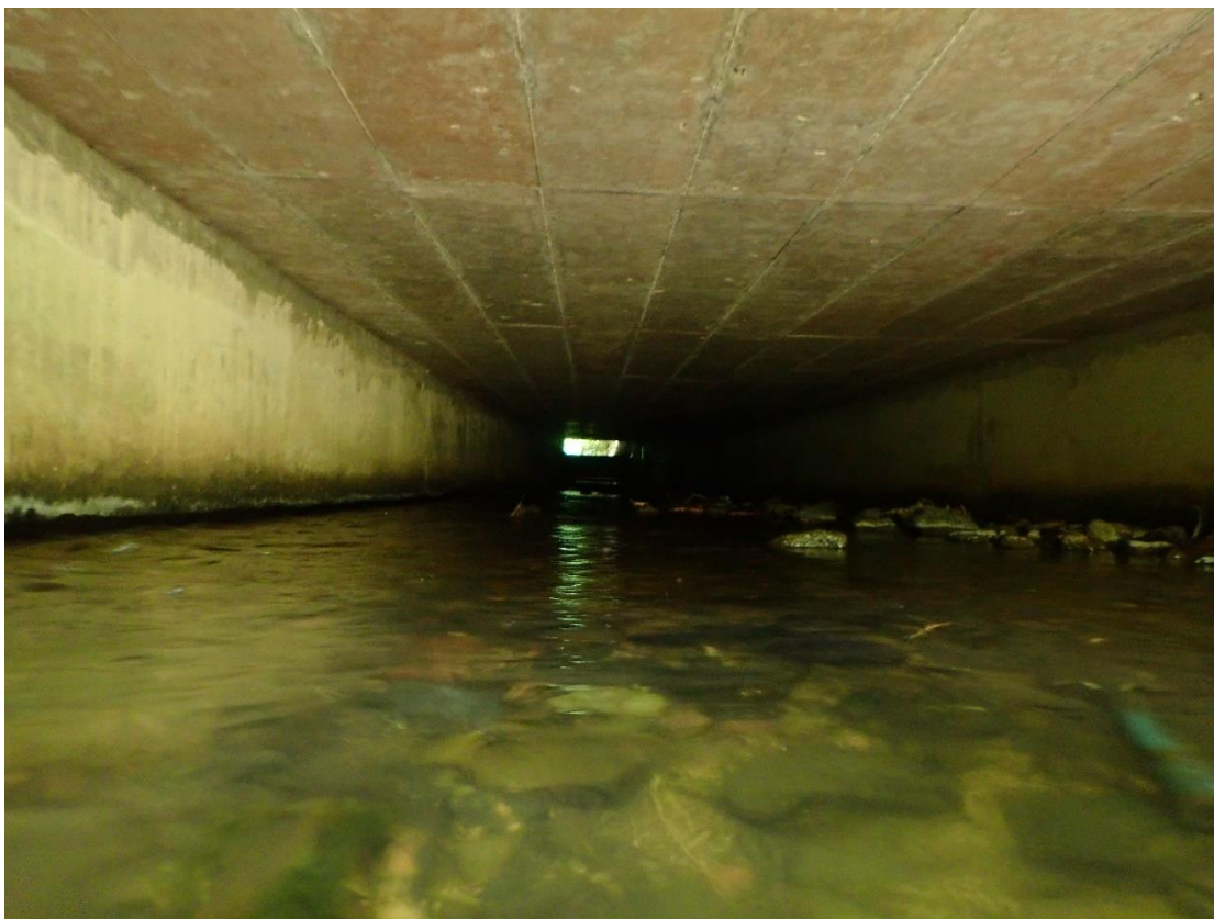
Plate 12: View looking upstream at channel of Loughlinstown River South as it flows under the N11 culvert.
