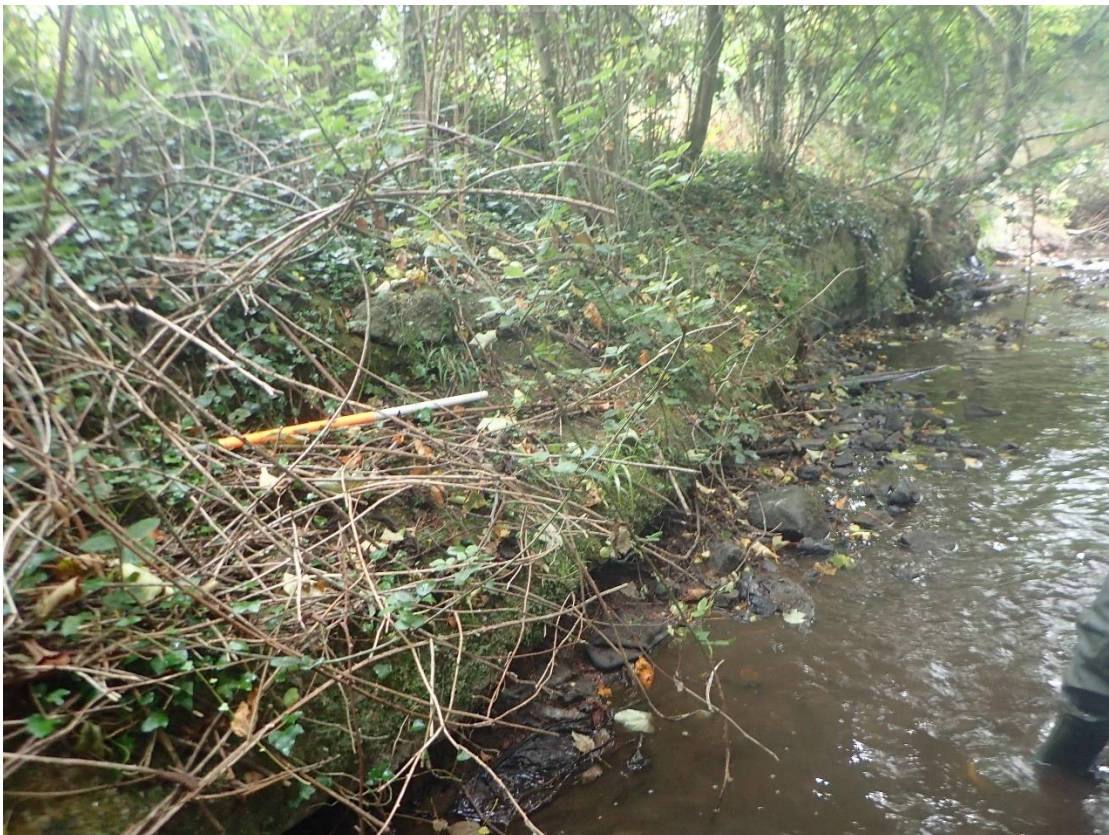
Plate 18: Clay slippage into river channel off left bank with stone retaining wall, ADCO 4, behind the slippage and extending downstream.
