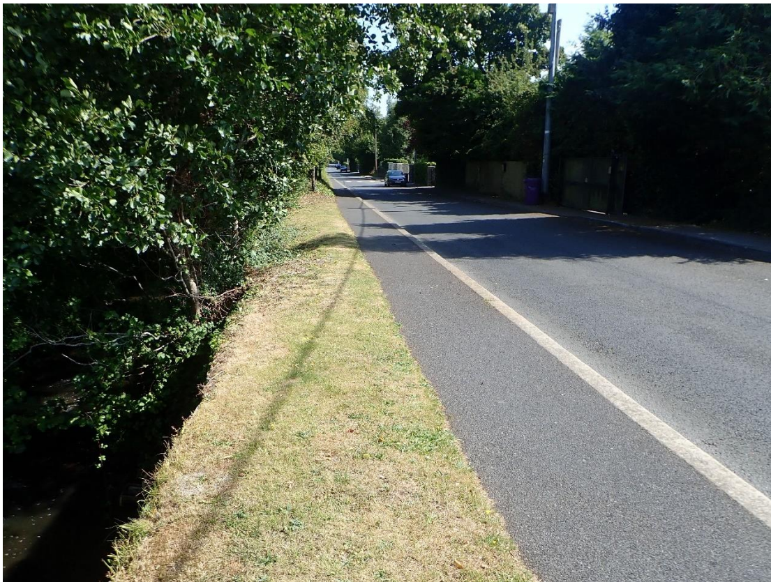
Plate 8: View east along Commons Road, where the top of the stone retaining wall is flush with the road surface that, in turn, serves as an embankment to the lower-lying properties on the other side of the road.
