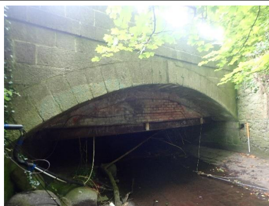
View from upstream looking at bridge arch ring and stone apron below
