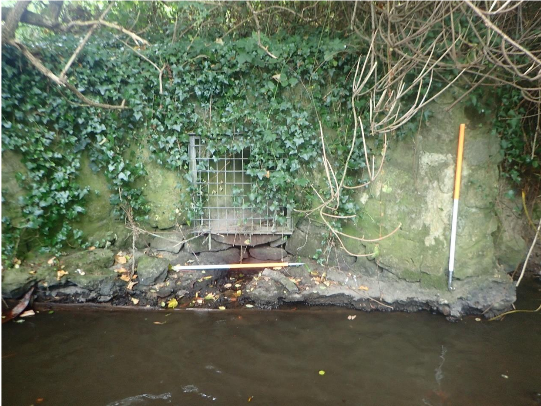
Plate 17: outfall pipe and attendant impacts on right bank, Loughlinstown River North.
