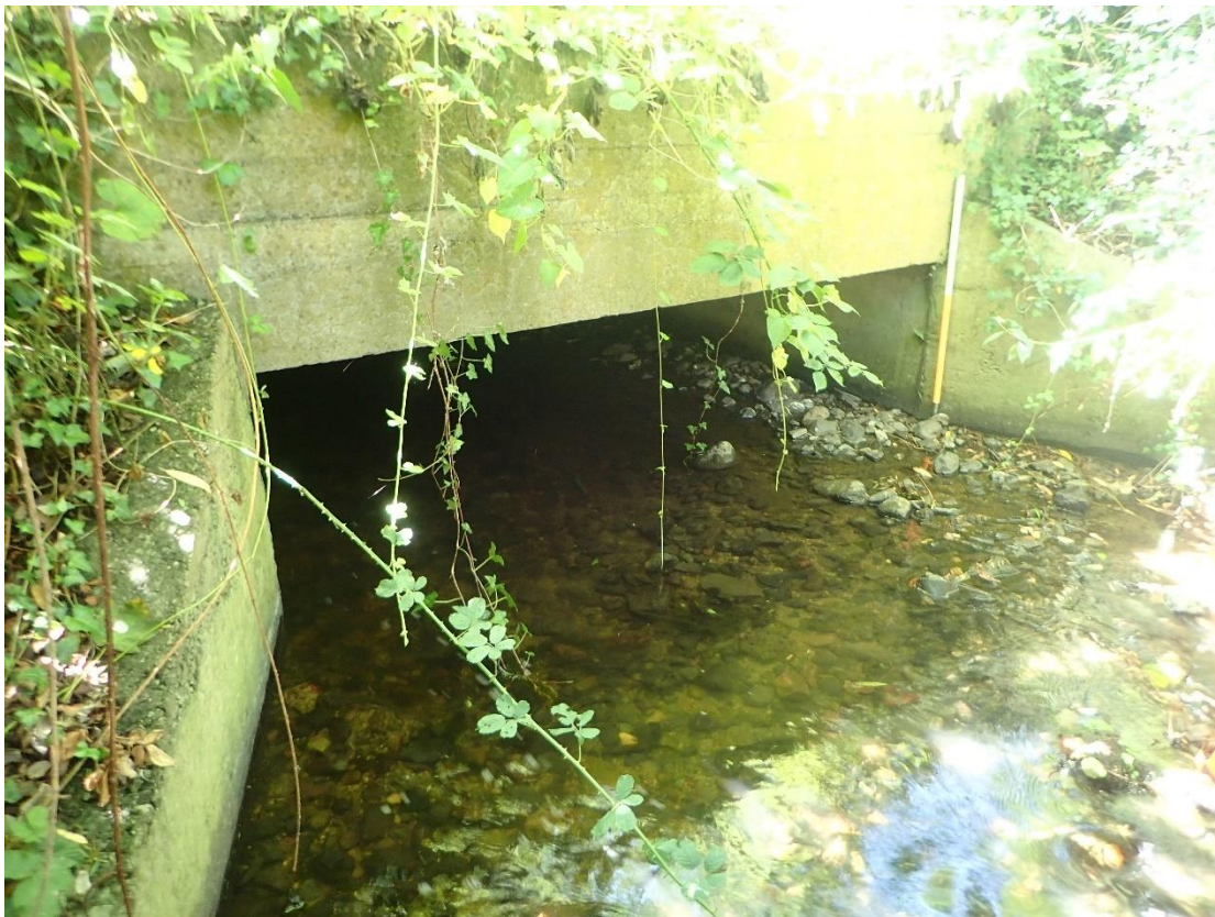
Plate 11: Current exit of the Loughlinstown River South on the east side of the N11 is through a reinforced concrete culvert.
