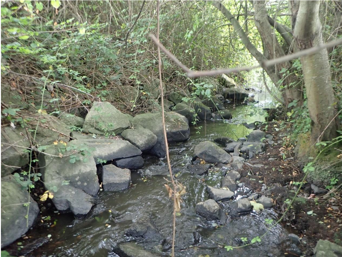
Plate 24: View looking downstream (east) along Carrickmines River, with rock armour boulder inserted at base of riverbank.
