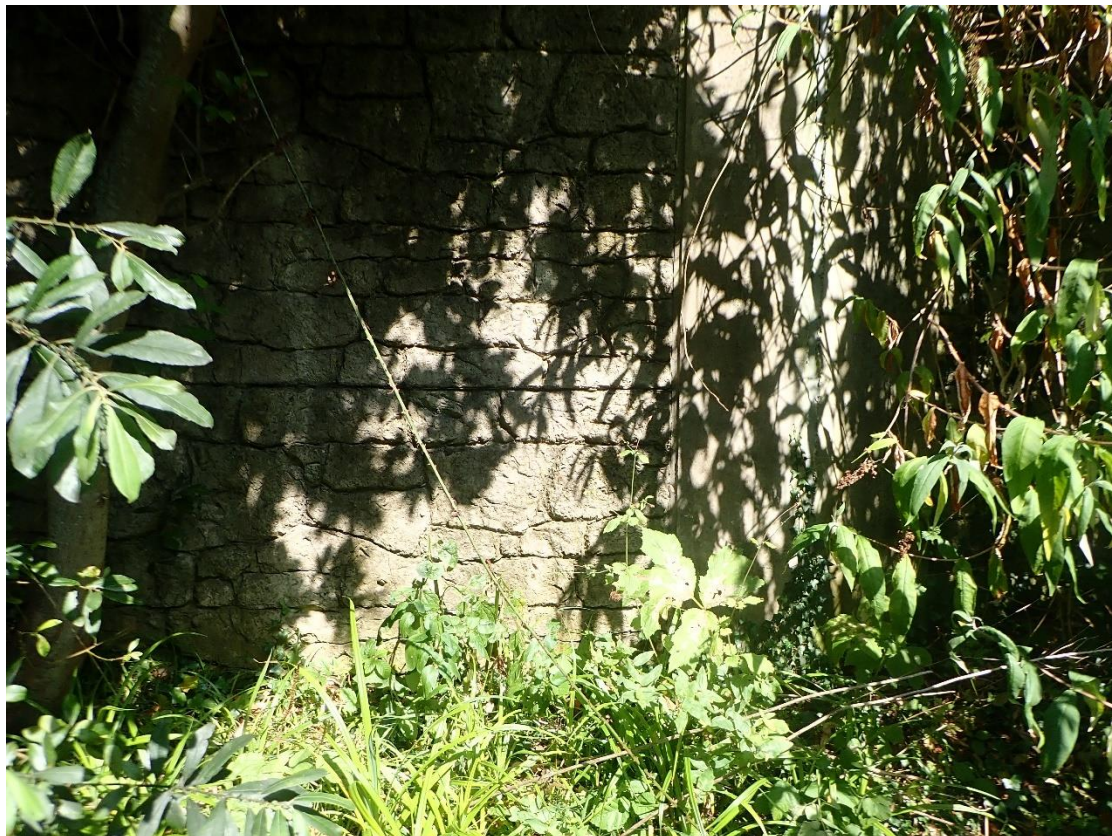
Plate 5: View of concrete slab retaining wall on left bank upstream of Shanganagh Bridge.
