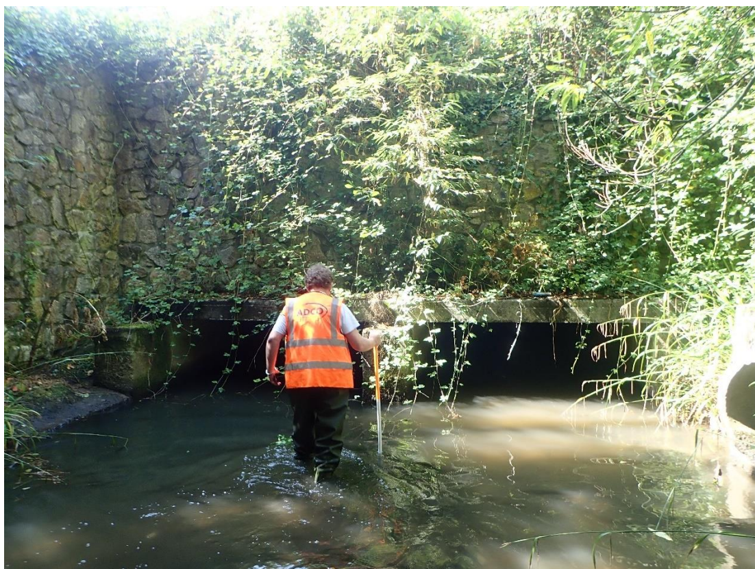
Plate 22: Current exit of the Loughlinstown River North on the east side of the N11 is through a reinforced concrete culvert.
