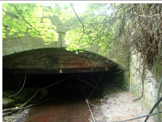
View from upstream looking at bridge arch ring and stone apron below. The bridge infill is sheathing to protect a later service pipe, supported on a steel girder
