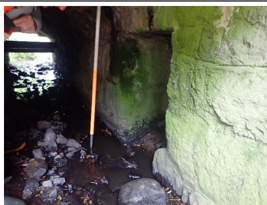
View of western culvert that empties into the southern arch from the south
