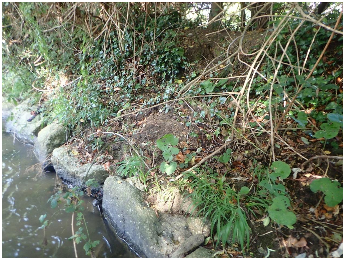
Plate 3: View of left bank showing rock armour protection added to base, downstream of Shanganagh Bridge.
