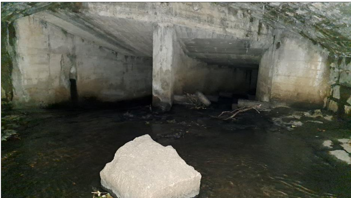
Plate 5.1 Example of a significant barrier to fish passage on the Carrickmines Stream at the N11 road culvert (high gradients under road & >2m fall)
