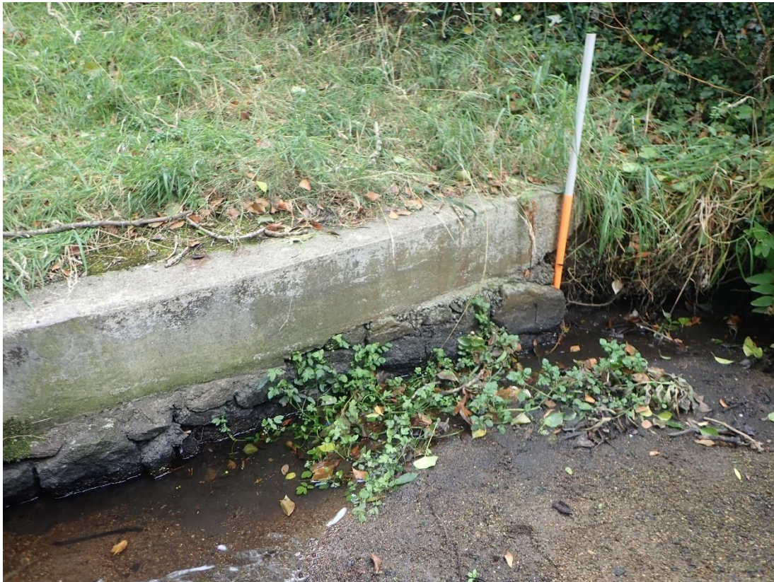
Plate 29: View of stone setting at base of streambank in Belarmine Park, where a modern reinforced concrete feature has been placed above it.
